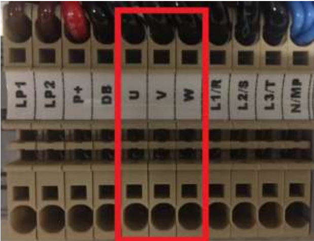
Figure 3- Motor Connection Terminals
